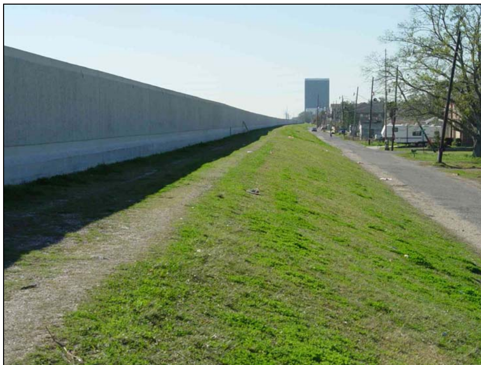
Figure 4.24 (lower): Concrete flood wall along the west side of the 17 th Street Canal in Jefferson Parish, where a street runs along the toe of the embankment. This scene is typical of the concrete I-walls constructed on steel sheetpiles driven into the crest of the drainage canal embankments in New Orleans in the 1990s to provide additional flood freeboard from hurricane-induced storm surges (photo by J. D. Rogers).
