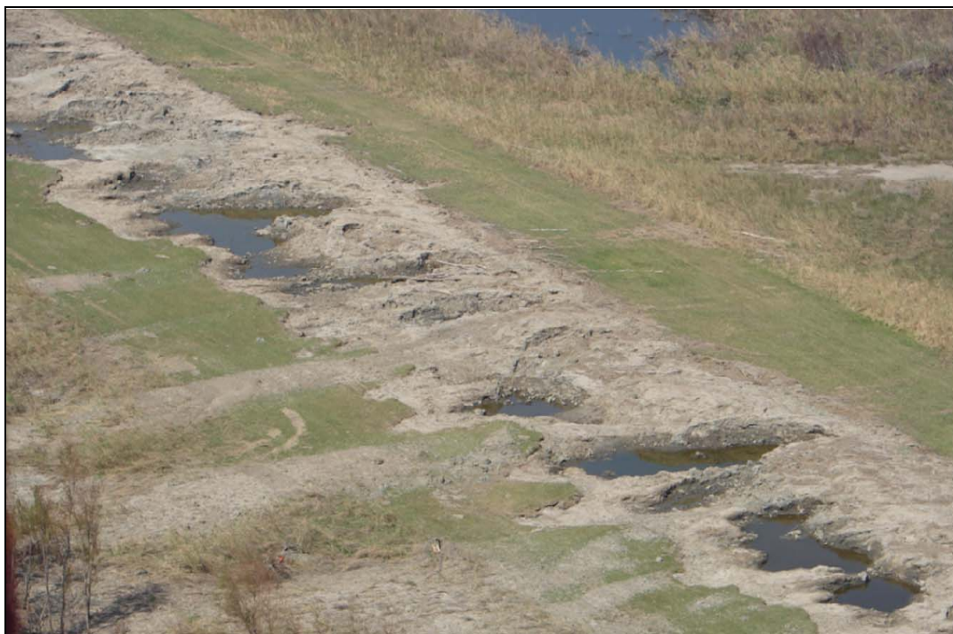
Figure 4.33: Area where the southwest bank of the MRGO channel levee within two miles southeast of Bayou Dupree was completely swept away by overtopping from Lake Borgne (photo by L. F. Harder).
