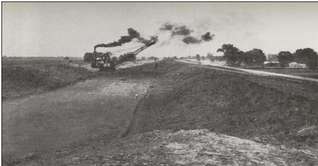
Figure 4.29: Mobile dragline constructing the Morrison-Picayuneville Levee about 25 miles south of New Orleans in June 1931 (from Elliot, 1932). Tower draglines could excavate materials up to a quarter mile away, dragging it back up onto the new levee.
