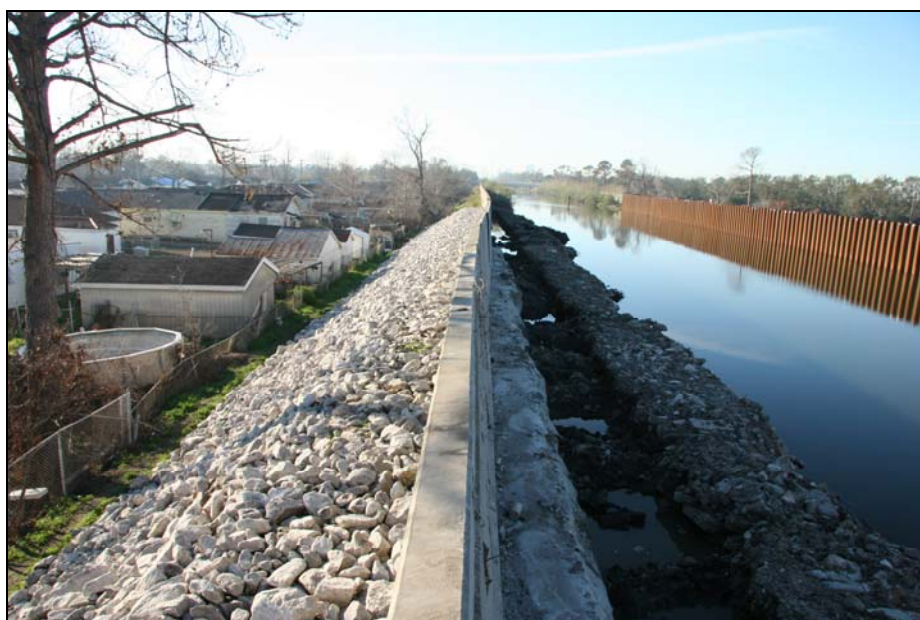
Figure 4.24 (upper): View looking up the east side of the London Avenue Canal near Robert E. Le Boulevard crossing showing the encroachment of homes against the slope of the levee. This situation was common across New Orleans (photo by C. M. Watkins).
